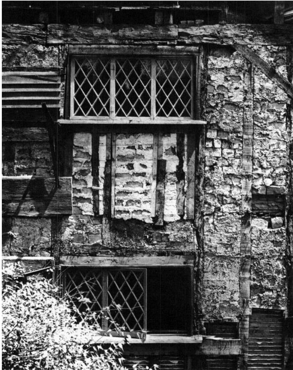
Whipple house repairs in 1953–1954 exposed the original frame with wattle and daub between the studs. Window sash with diamond panes was installed in 1898 during restoration. Photo by Peter Zaharis.
